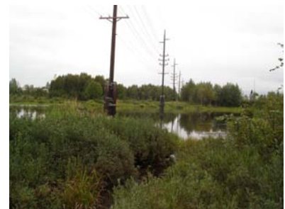
CEA transmission line crossing Tina Lake.
